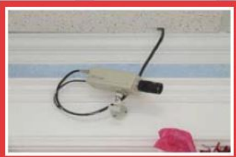
Interior Camera Installation
