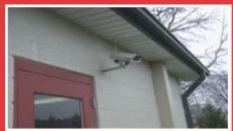
Exterior Camera Installation
